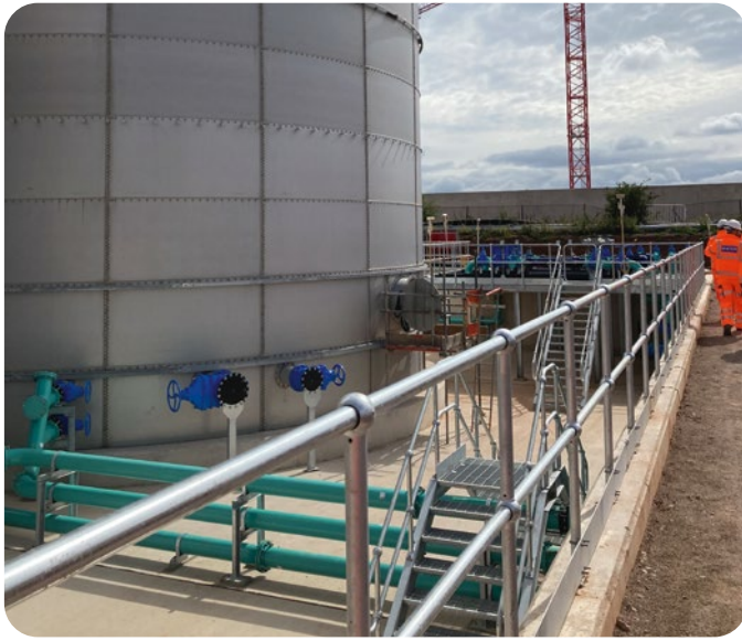
Wanlip Sewage Treatment Works, Leicestershire
